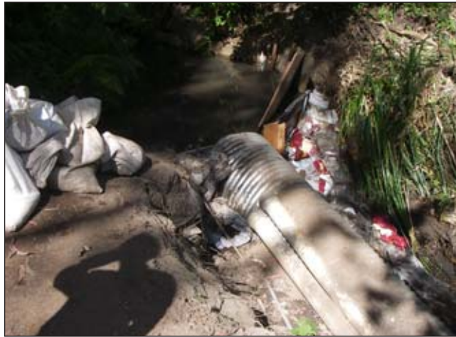
PHOTO 11: Point of Diversion on San Vicente Creek.
