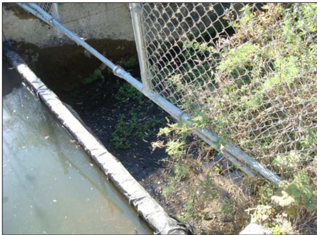
PHOTO 31: Spill over from Denniston Reservoir into Denniston Creek.
