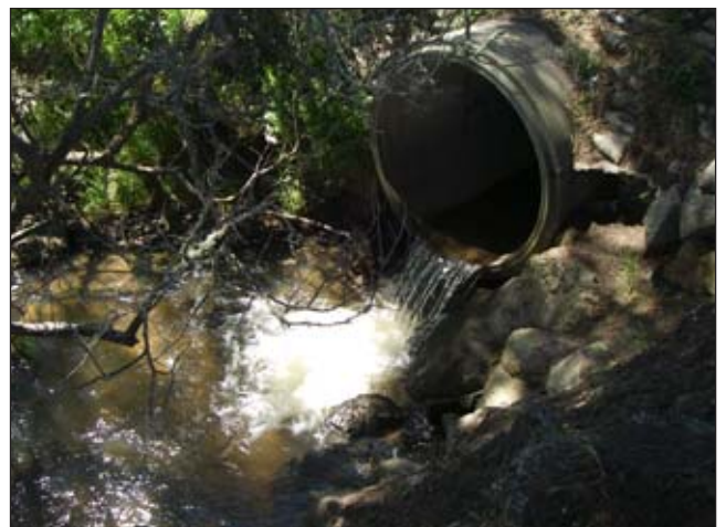
PHOTO 19: Possible barrier on Denniston Creek.
